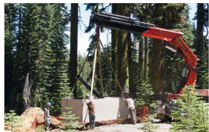
Bailey Construction easily sets this precast vault that will be topped with a restroom shelter using their PALFINGER PK 150002 H
