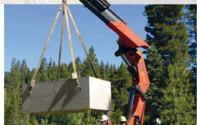
For this job, the PALFINGER PK 150002 H will extend out approximately 28' to set a precast concrete vault weighing 17,800 lbs.
