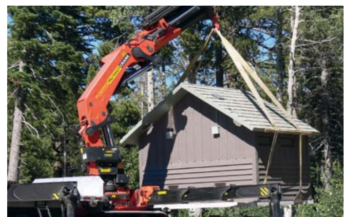
This may not look like a heavy load but restroom shelters such as this one are now entirely concrete and can weigh up to 49,000 pounds each
